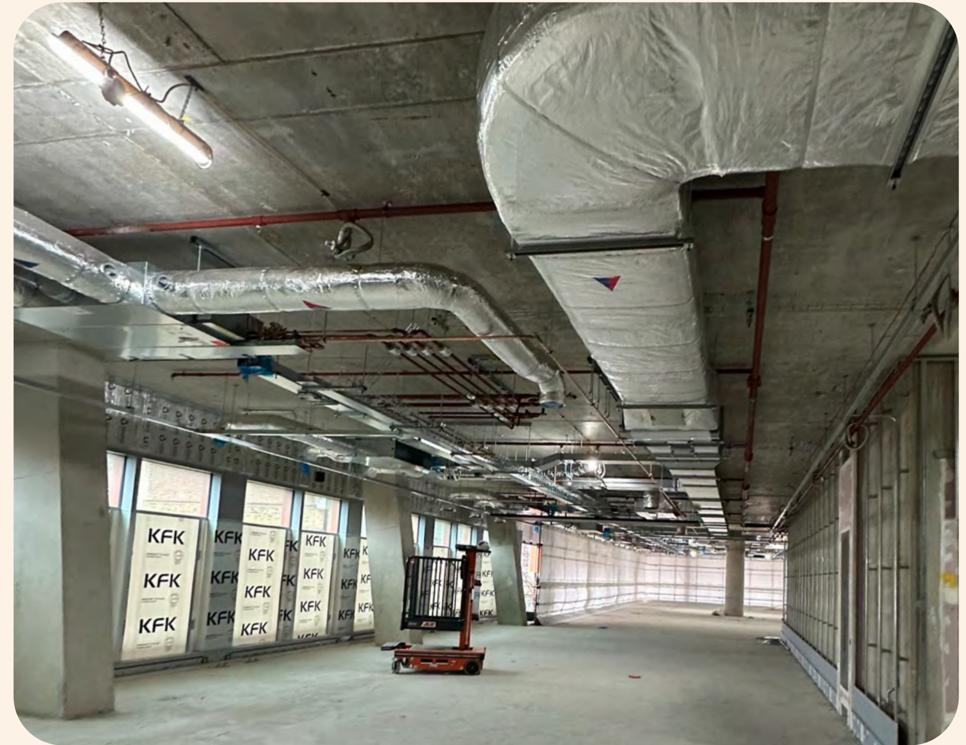
Level 2 - Exposed Services
