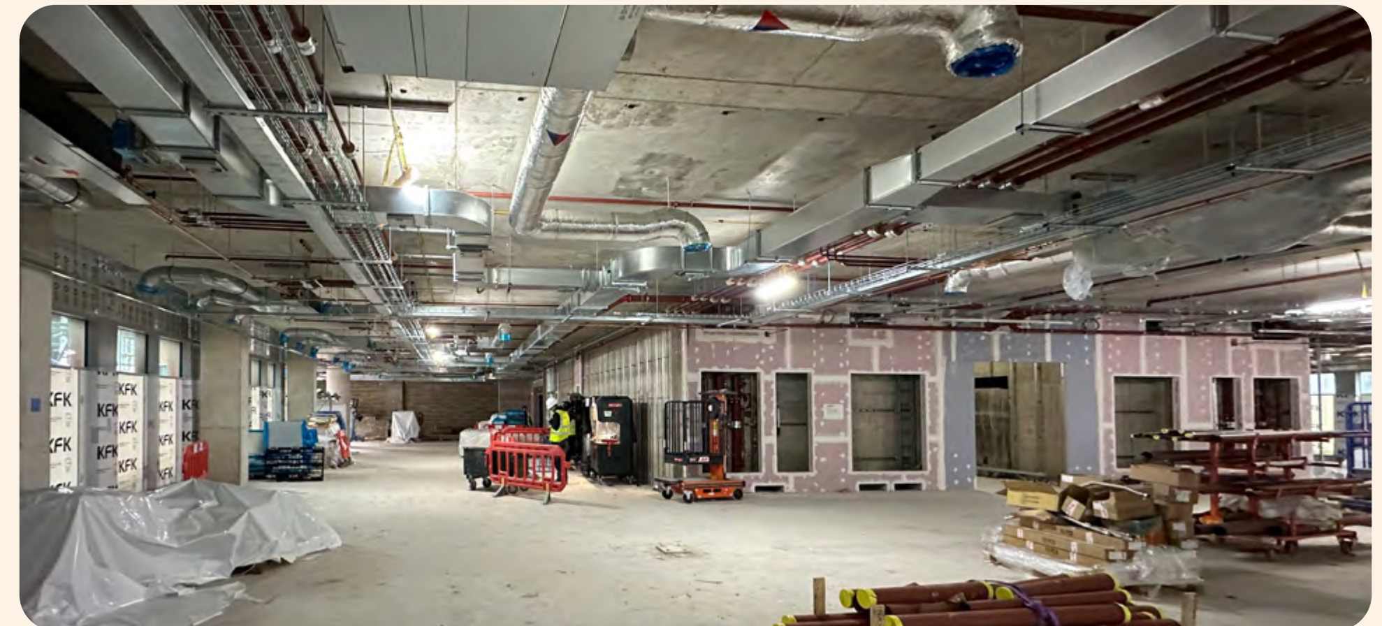
Level 2 - Exposed Services
