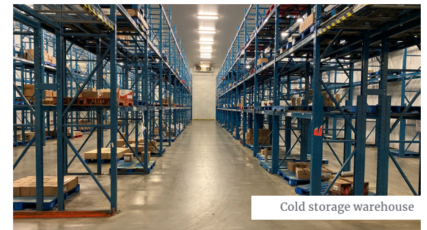
Cold storage warehouse
