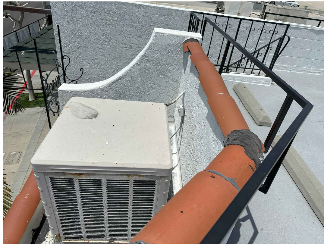
View of HVAC Unit Facing E. Coast Hwy.
