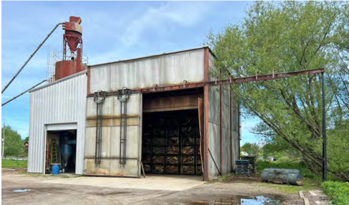
Bldg. 4: 1,749± SF Boiler/Kiln Facility With 12'W x 14'H Overhead Door & Dual Sliding Doors Opening 15'6"W To 31'W x 20'H
