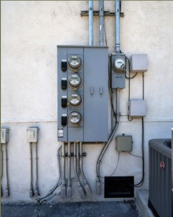
New main and sub panels
