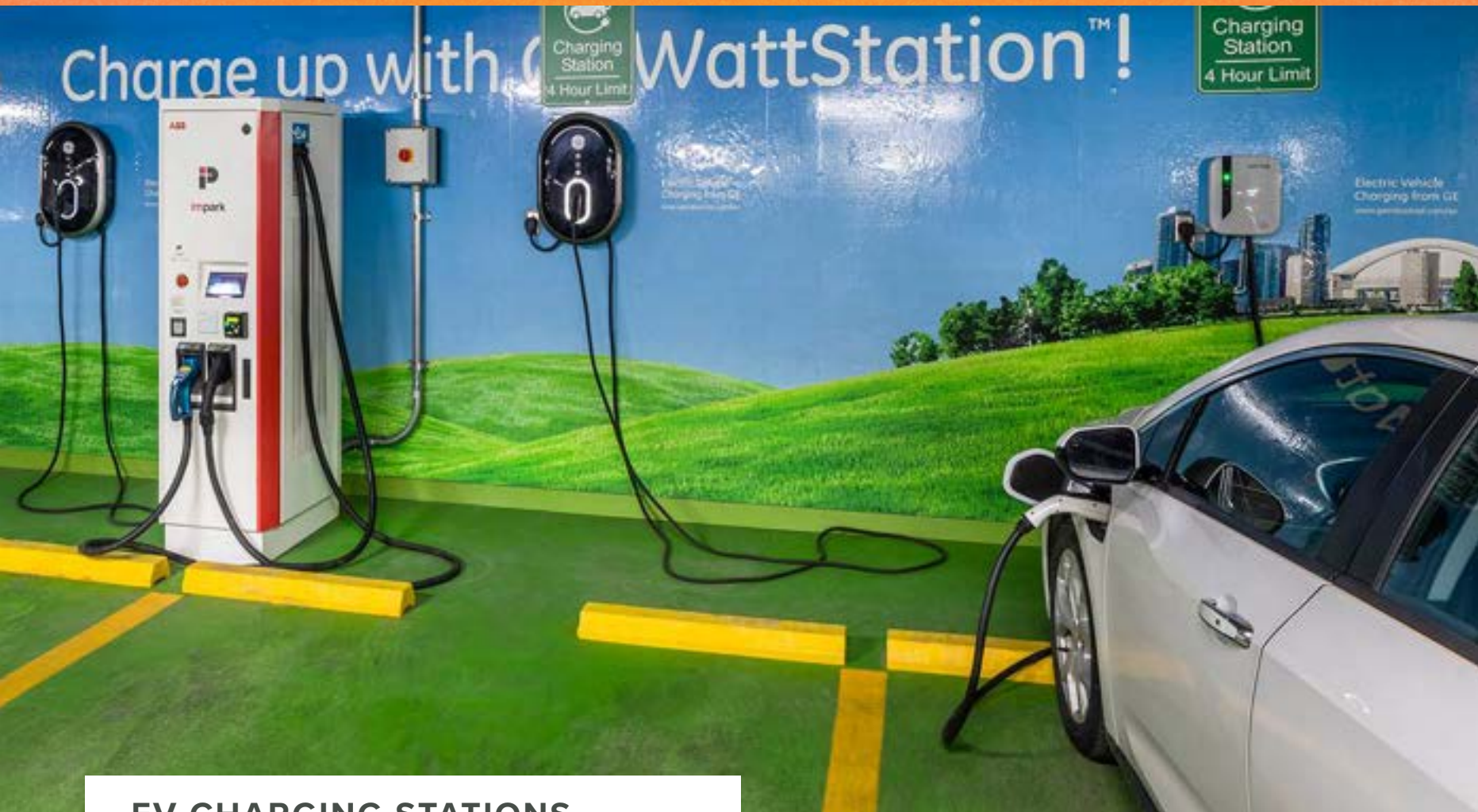
EV CHARGING STATIONS
