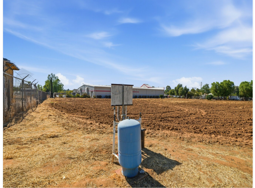
Well Access tank/pump
