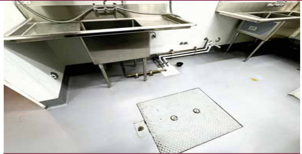
In-Ground Grease Interceptor
