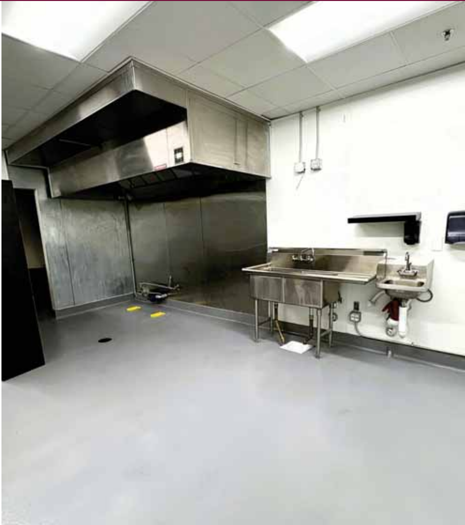
Type I Exhaust Hood 11' with Ansul Fire Suppression System
