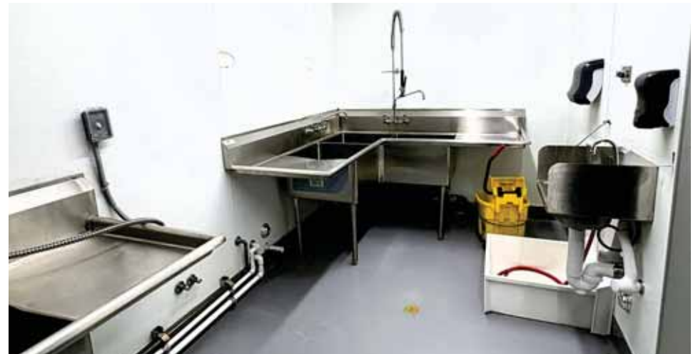
Stainless Steel Compartment Sinks and Mop Sink
