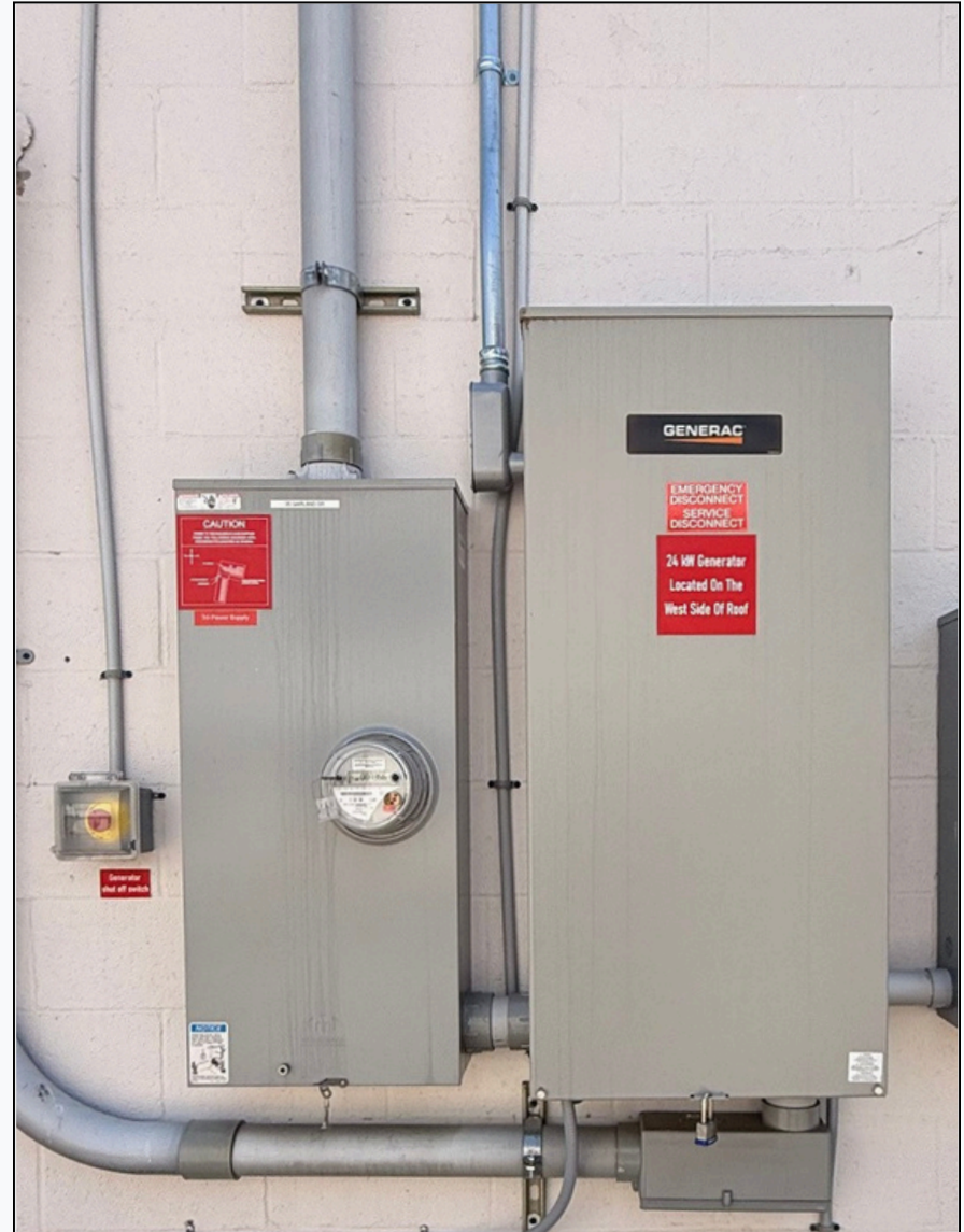
24KW Generator Provides Backup Power
