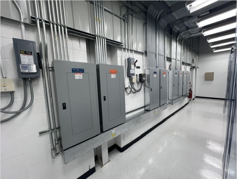
Electrical distribution panels
