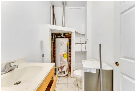
FRONT HALF BATH — HOT WATER HEATER
