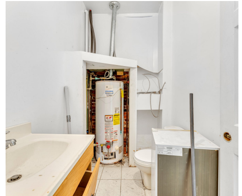
FRONT HALF BATH — HOT WATER HEATER
