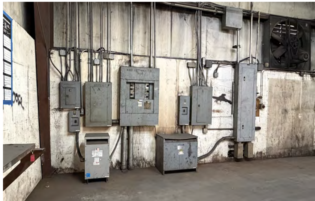
Heavy 3-phase Power
