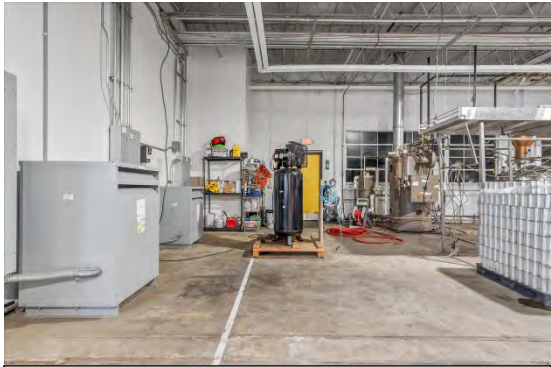
View of Inside Power
