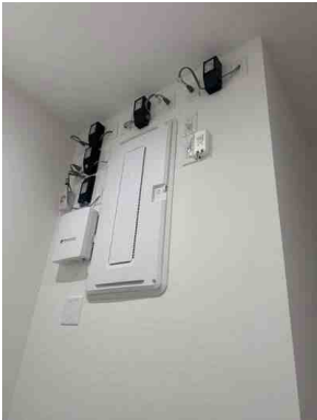
smart system control center
