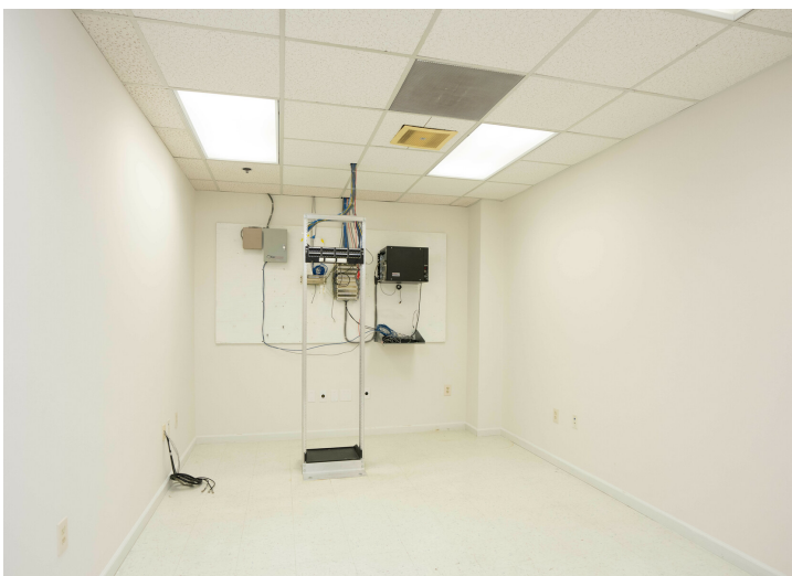
Dedicated Server Room
