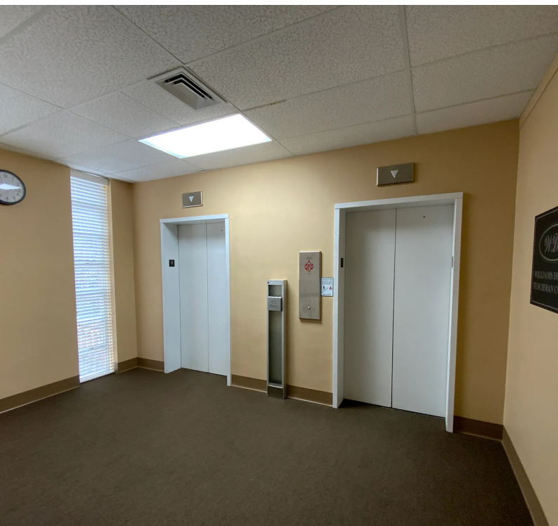
2 Recently Renovated Elevators Basement to 8th Floor
