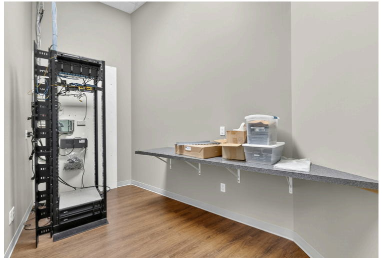
Designated Server Room
