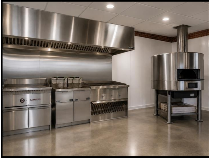
Kitchen; Newly Installed Range Hood & Rotary (multi-use) Pizza Oven
