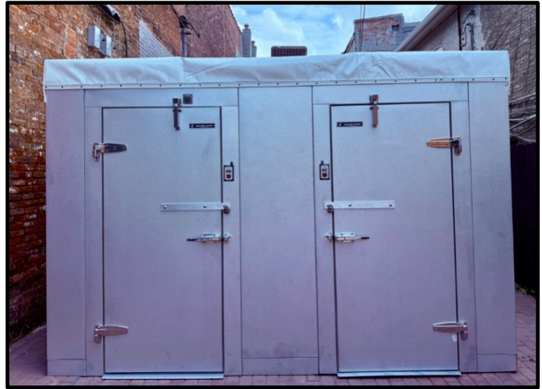
Exterior: 12x12 Walk-in Refrigeration & Freezer
