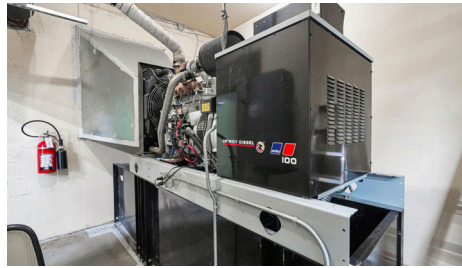
BACKUP GENERATOR ROOM
