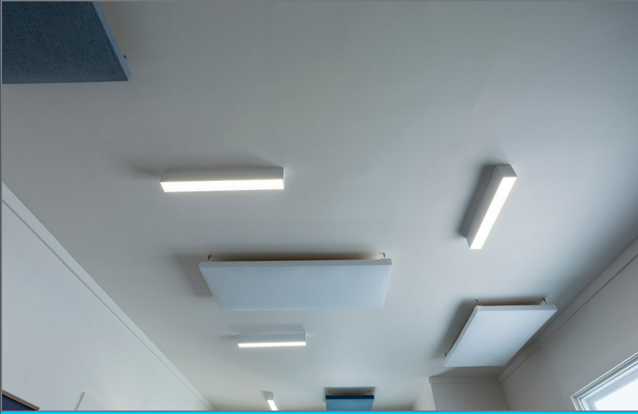
LINEAR LIGHTING WITH ACOUSTIC TREATMENT
