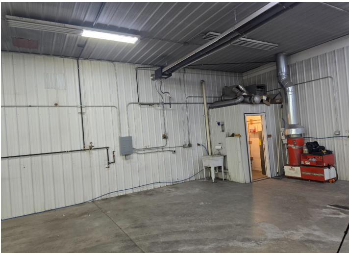
PLUMBED FOR AIR
