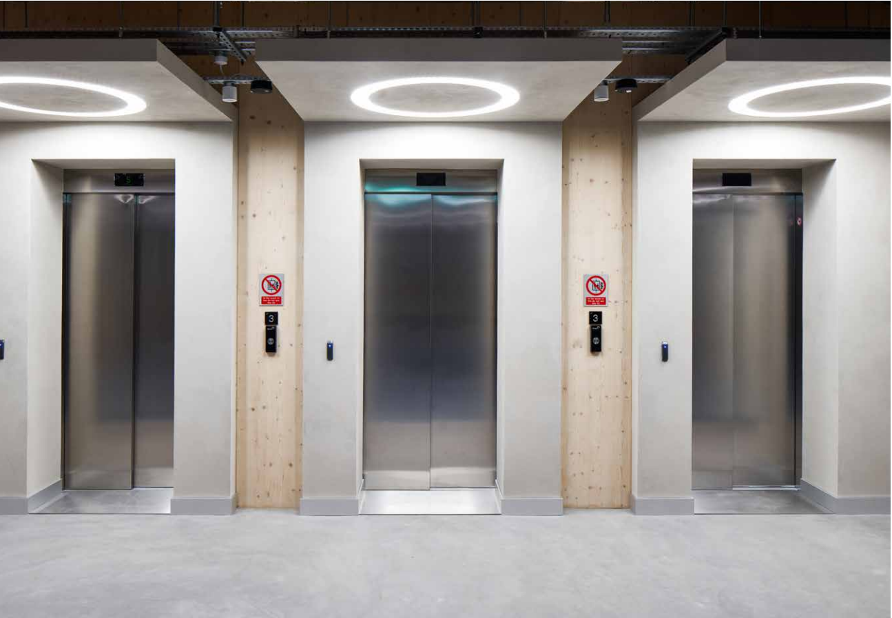
x3 passenger lifts
