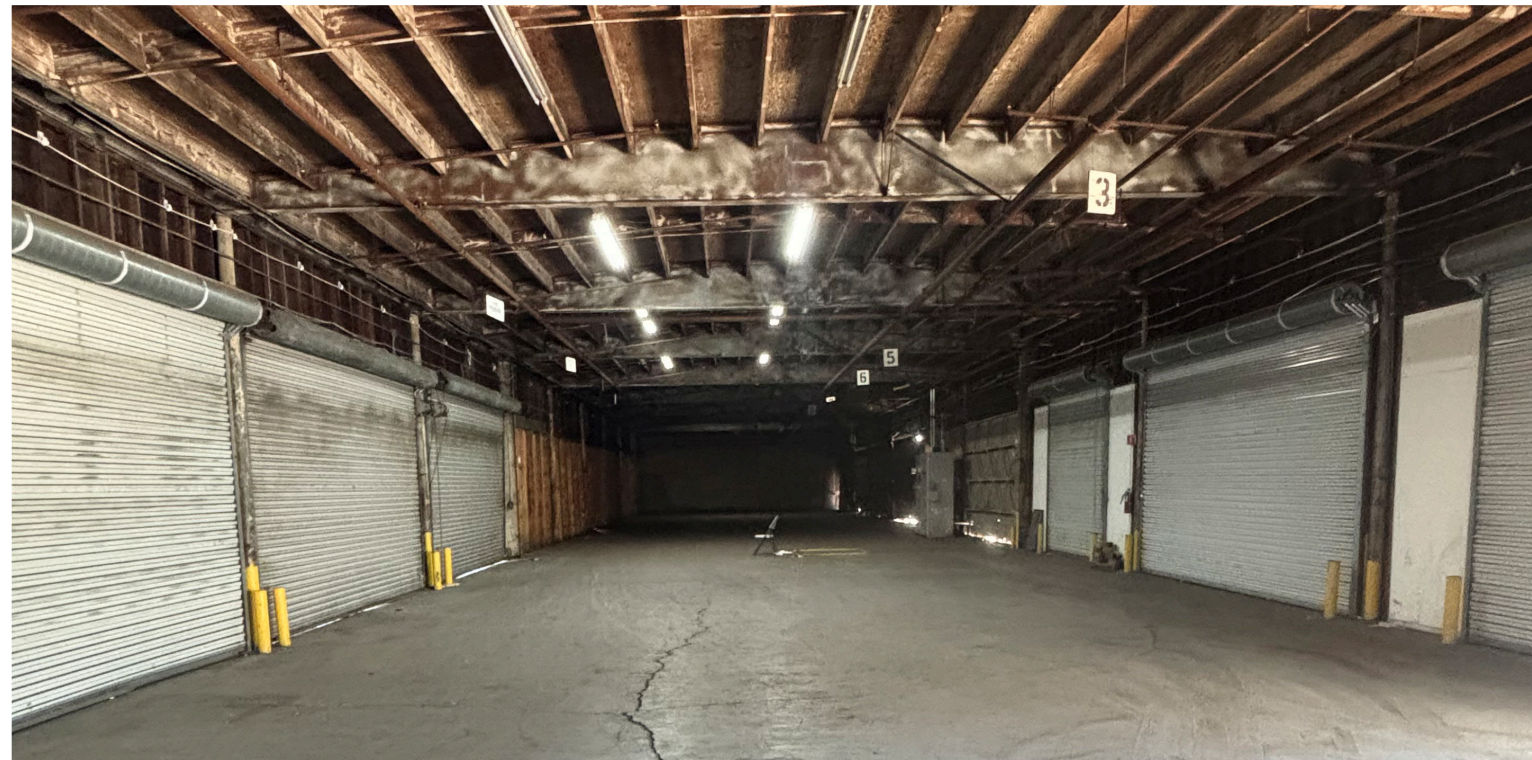
Interior of Cross-Dock (14' Clear)
