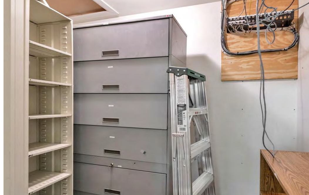
IT Room in Front Building
