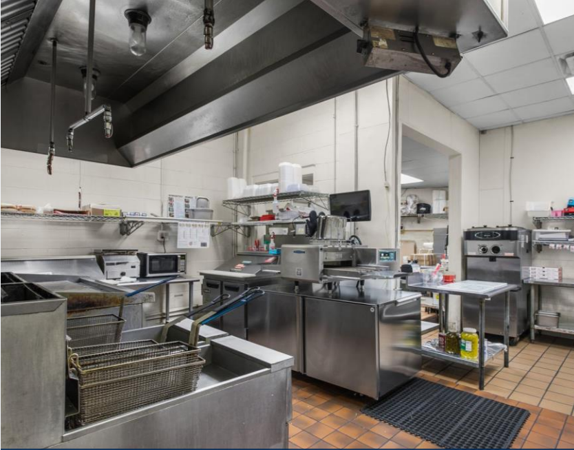
Commercial Kitchen & Hood System
