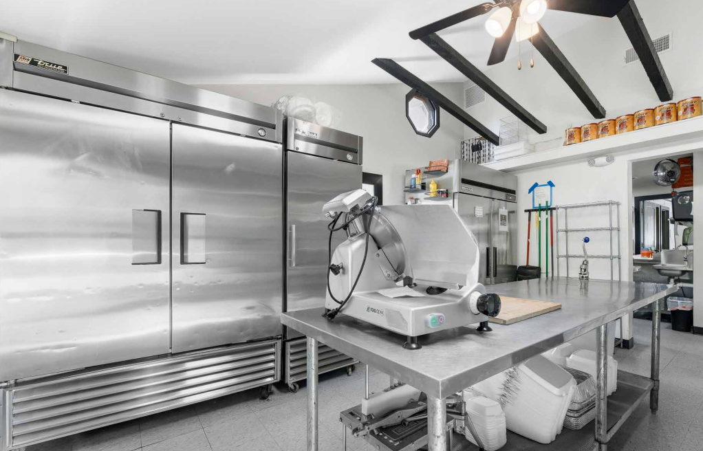
Restaurant Commercial Kitchen.
