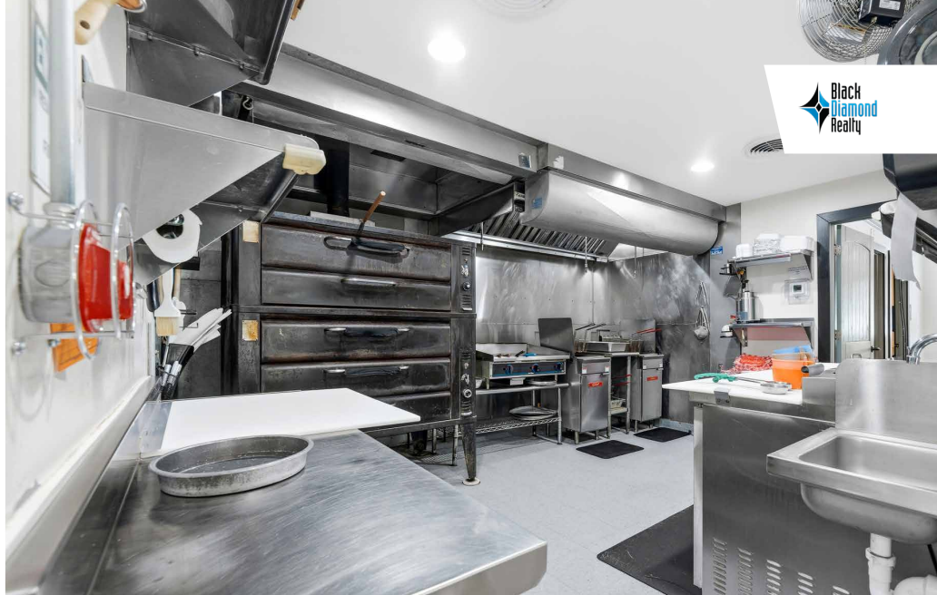
Restaurant Commercial Kitchen.
