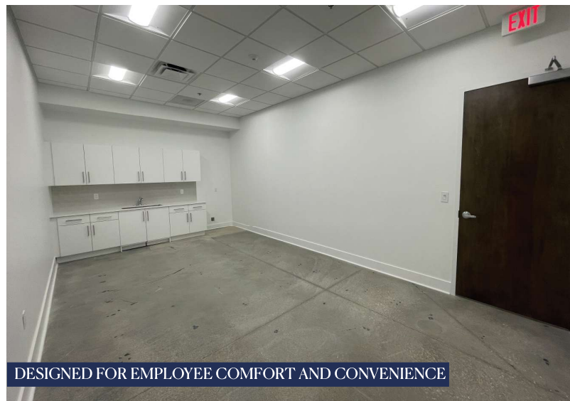
MODERN KITCHEN WITH WAREHOUSE ACCESS DOOR
